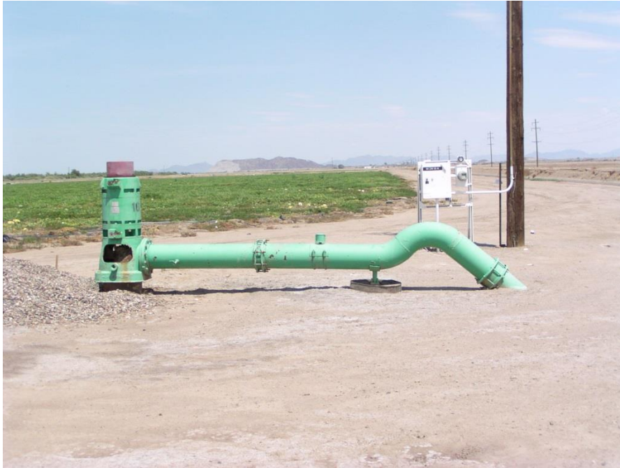
Figure 3.14 Drainage Well within the WMIDD
