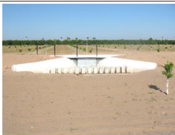
Figure 3.6b High Flow Irrigation Turnouts
